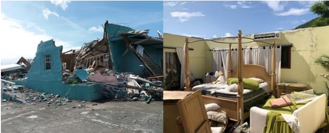
Completely uninhabitable homes after the strong winds associated with Irma and Maria.
